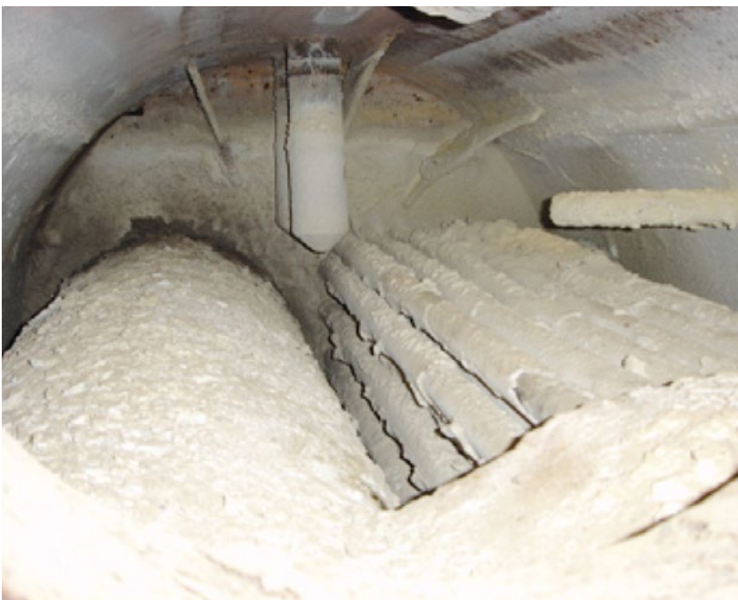
Figure 1: A lack of water treatment caused the formation of a hard layer which can lead to boiler explosion in the extreme case.
