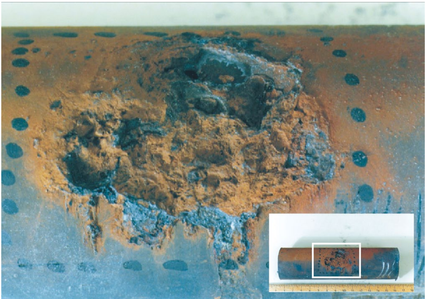
Figure 3: Oxygen attack on a cut-out smoke tube
