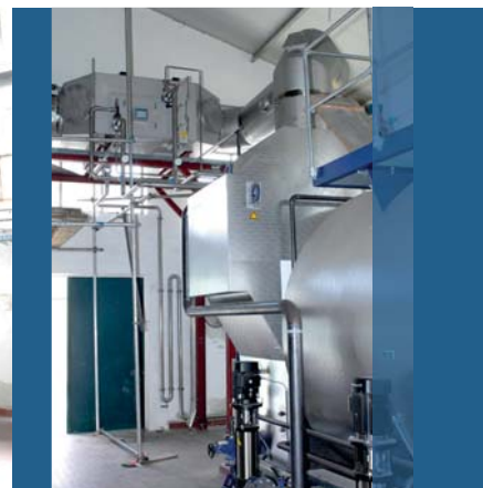
System with economizer for feed water preheating and condensing economizer for preheating of brewing water connected in series
