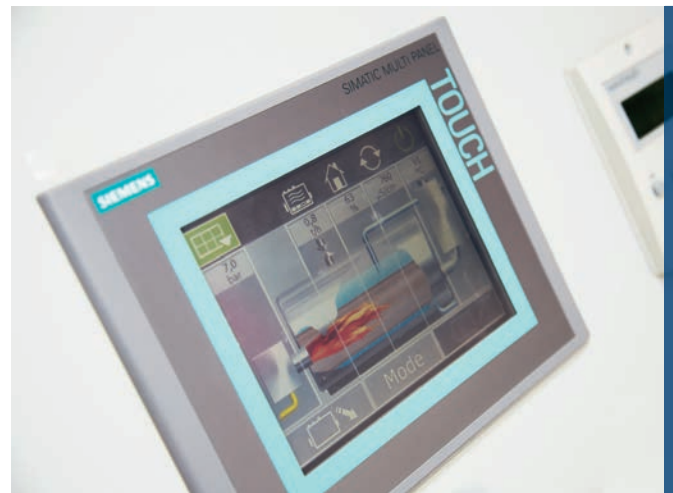
The excellent data transparency of the boiler control enables operation to be optimised
