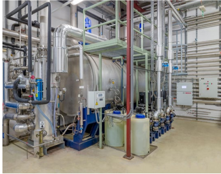
The vapour cooler and the heat recovery and expansion module for desalting water supplement the existing feed water deaeration system.
