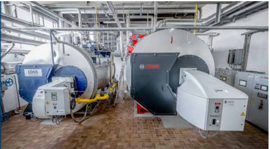
For efficient and flexible use: The two steam boilers UL-S at the NÖM dairy.
