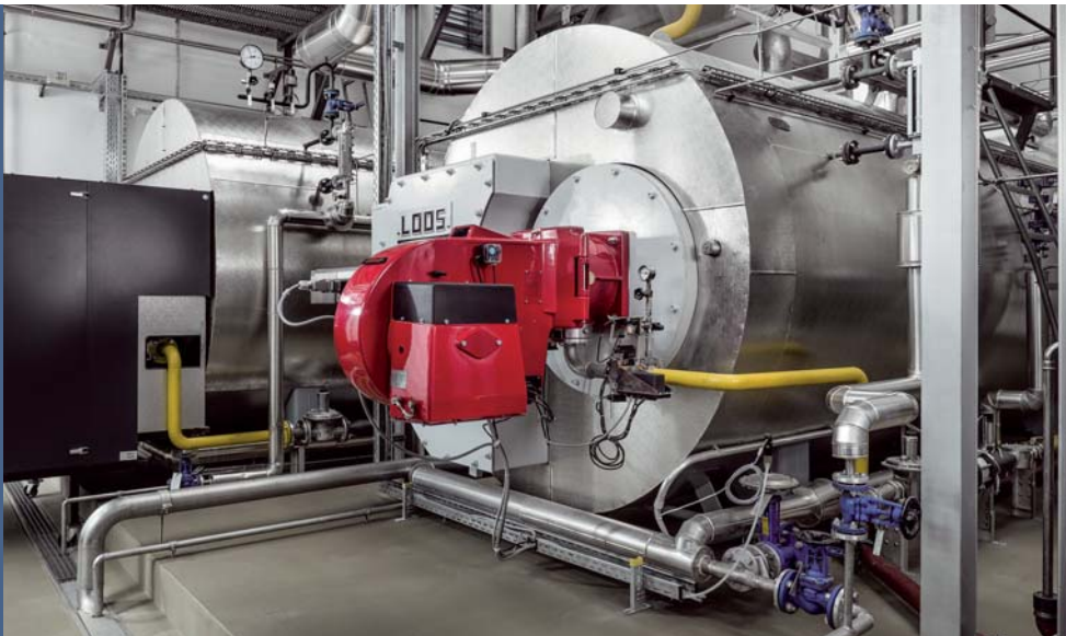
The modernised steam boilers with oxygen and speed-controlled natural gas burners at Oettinger Brauerei.
