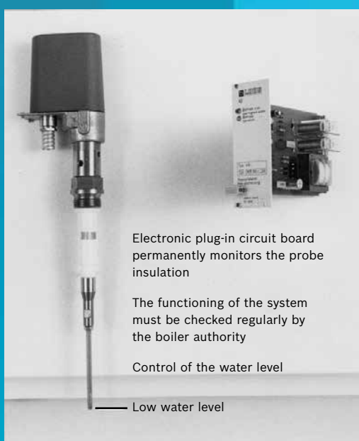
Figure 3: Two-channel probe water level monitor – the operation of the system must be checked regularly by the boiler inspection authority
