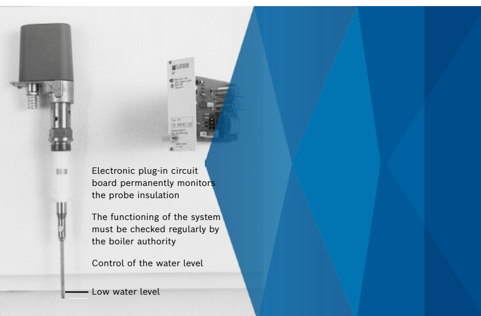
Figure 3: Two-channel probe water level monitor – the operation of the system must be checked regularly by the boiler inspection authority
