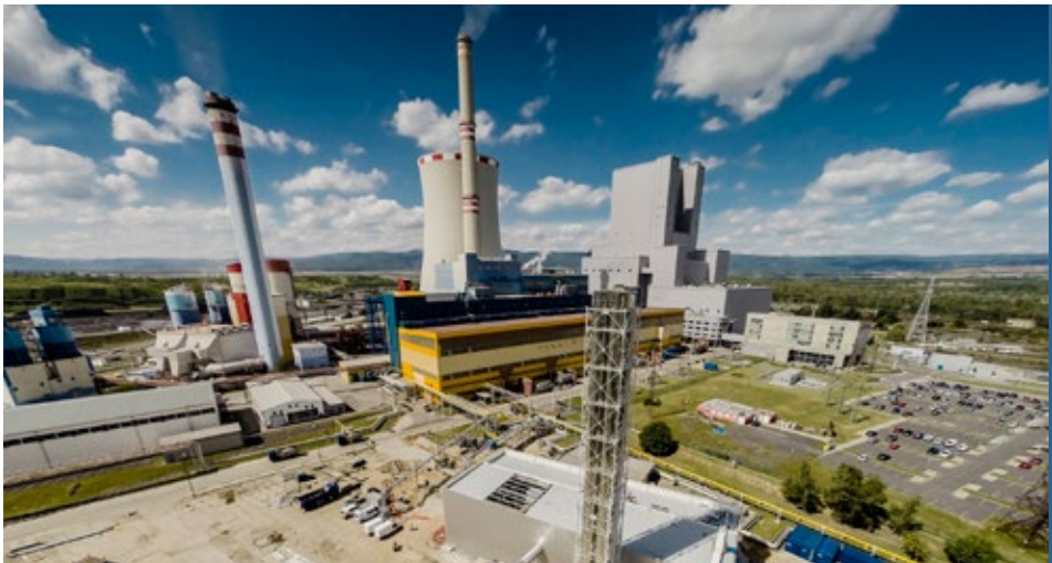
Ledvice power plant during the building phase of the new boiler house
