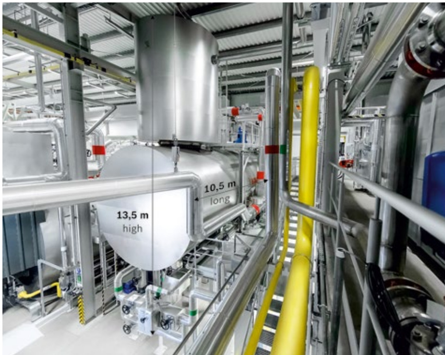
Bosch's huge feed water system with a deaeration capacity of 177 500 kg/h can store up to 100 000 litres of feed water
