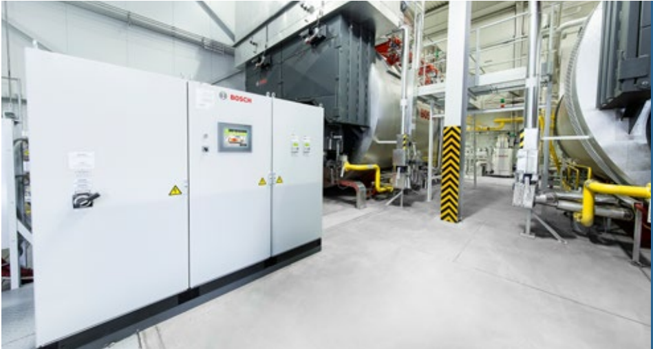
Intelligent control concept for automated boiler operation
