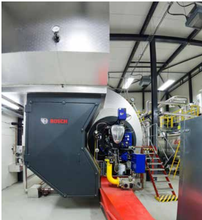
The UL-SX steam boiler ensures stable power plant operation.
