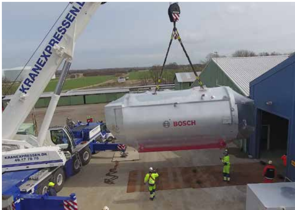
Pictures: Lifting into the boiler house, installation and commissioning of the UL-SX steam boilers.
